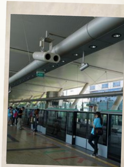
Dover MRT station's platforms are situated on both sides of the train tracks
