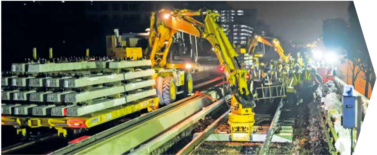
Sleeper replacement work currently underway on the NSEWL and will be completed by 2016.
