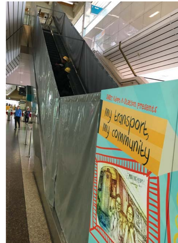
We are upgrading our escalators to serve commuters better.
