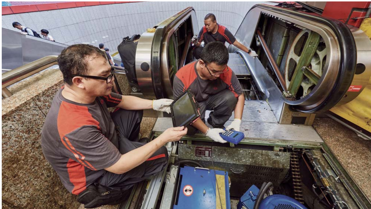
Staff utilising MOMS for escalator maintenance.
