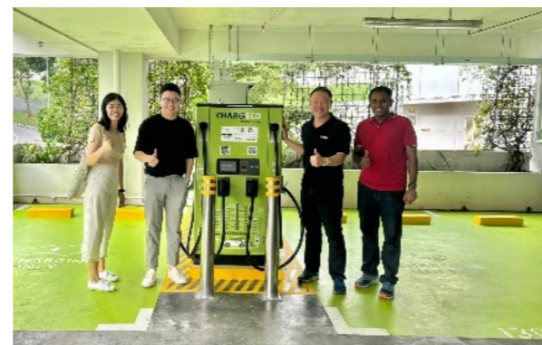
ChargEco at Republic Polytechnic
