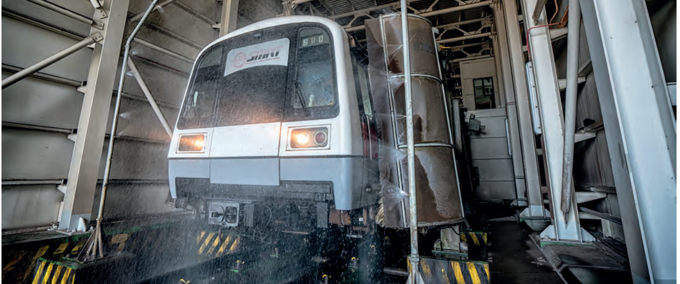
Train washing plant includes a water recycling system.
