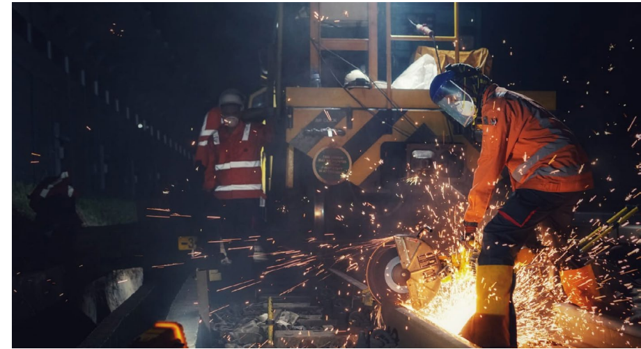
We invest significant effort in renewing and upgrading our tracks and trains to enhance reliability and service for commuters.
