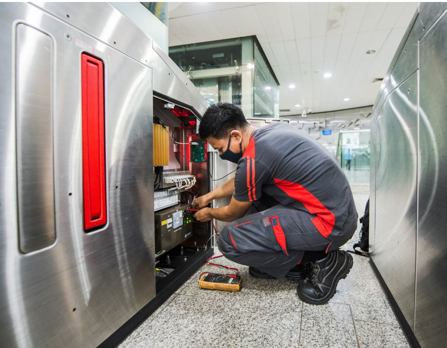
Strides Engineering offers end-to-end rail-related services including the designing, planning, implementation and operation of Automatic Fare Collection gates.
