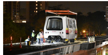
Work is underway to renew and replace the Bukit Panjang Light Rail Transit, to enhance its safety and performance.
