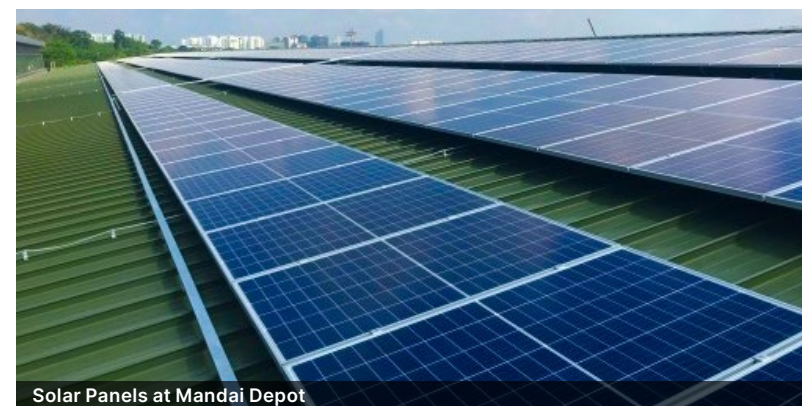
Solar Panels at Mandai Depot
