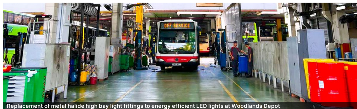
Replacement of metal halide high bay light fittings to energy efficient LED lights at Woodlands Depot
