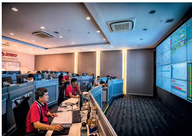
Together with our Operation Control Centre, SMRT Trains' new Maintenance Operation Centre (MOC) monitors the NSEWL 24 hours a day.
