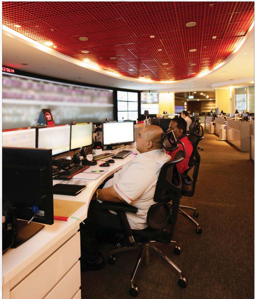
The Operations Control Centre (OCC) for the NSEWL and CCL, located at Kim Chuan Depot.
