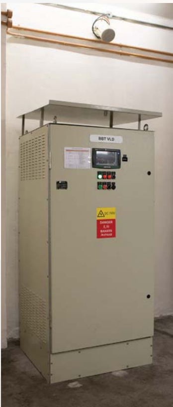
Voltage Limiting Device to isolate faults to a limited sector of a track.
