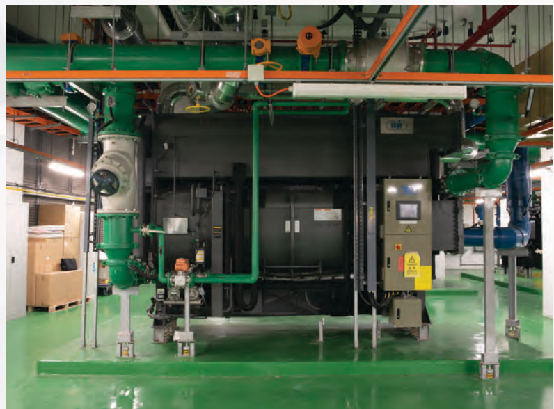
Solar adsorption chiller that provides additional cooling capacity to the Depot.
