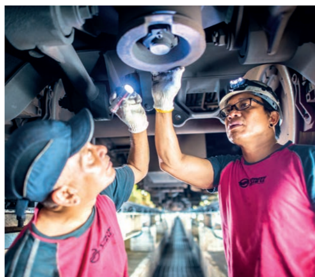
SMRT Trains' maintenance crew carry out regular checks on train air conditioning units to ensure you have a comfortable journey.
